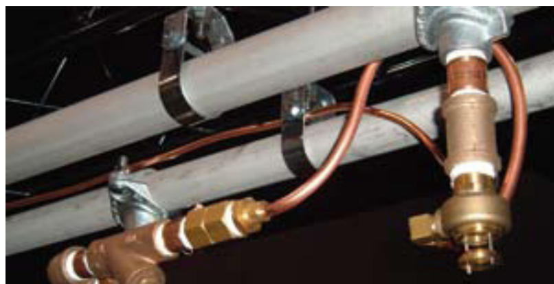
Emitter and Piping
