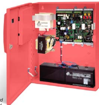
Cabinet with option card and batteries installed.
